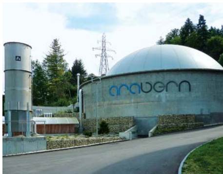
Biogas measurement for the supply of a combined heat and power plant, ara region bern ag, Switzerland
